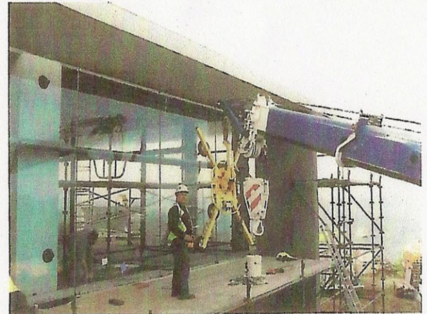
Laurie Patterson placing 25 mm, 600 kg glass into frames using the remote control. The working space was 10 mil.
