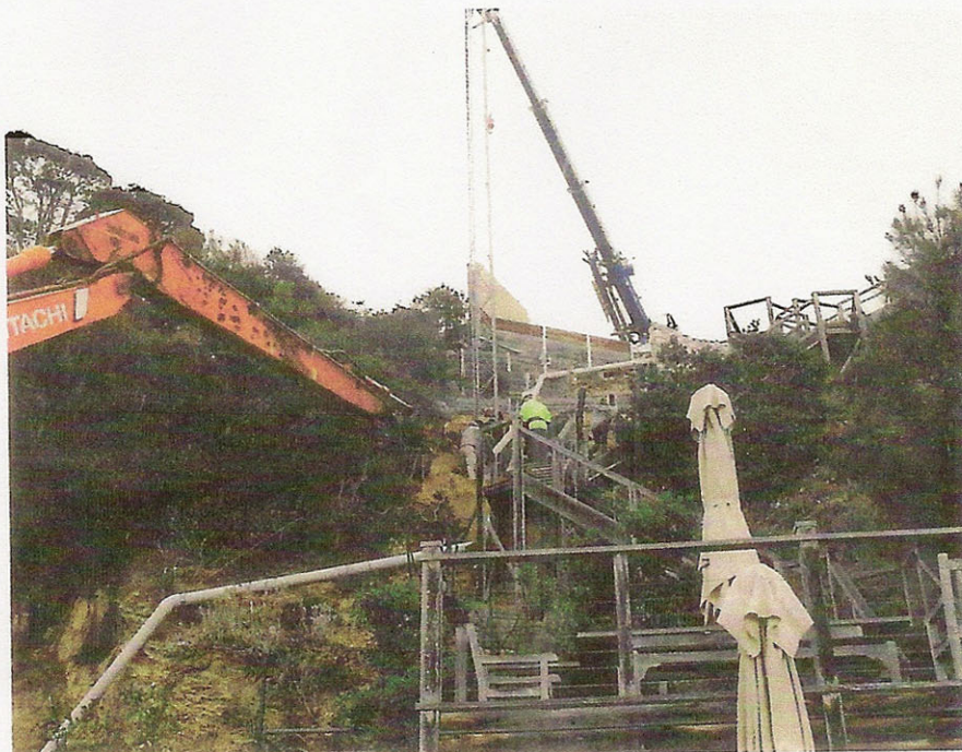
Truss suspended from Demag AC 25 at the top of the cliff, with excavator at the base providing hydraulic power for the auger attached to the truss.
